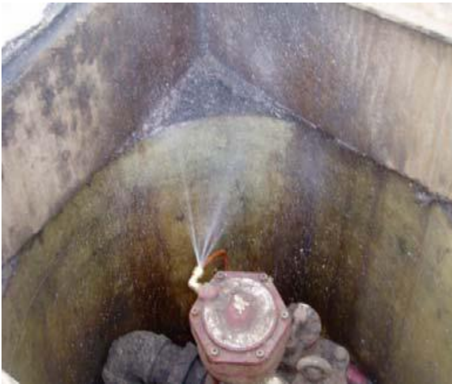
Leaking Line Leak Detectors
