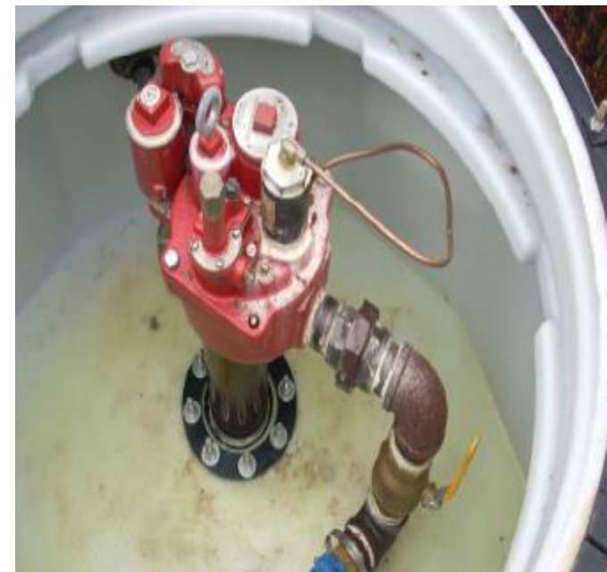
Red Jacket STP in Sump
